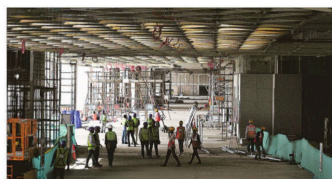
(Top) At Vihari in Mumbai, one of the many tunnels through which the Mumbai-Ahmedabad high-speed line will pass, work on at the Ahmedabad station of the bullet train
